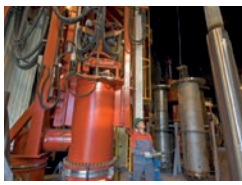
Melting & Remelting HPS
